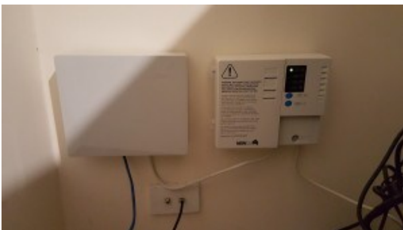
NBN Connection box with cover taken off
